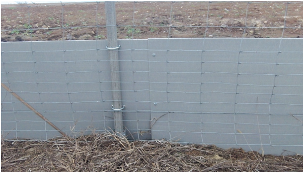
Fig. 3. Glass Fiber Reinforced Polymer (GFRP) plates used as barrier for preventing vehicular turtle mortality at the "Trakiya" motorway. Note the stable mounting of the plates to each other and to the metal pole
