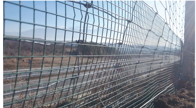
Fig. 4. Close-up of the fences constructed at Lot 1 of the Struma Motorway. The fine net is buried deep in the substrate and firmly fixed at the basis of the standard rabbit fence
